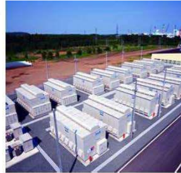
204 MWh NGK battery in Japan
