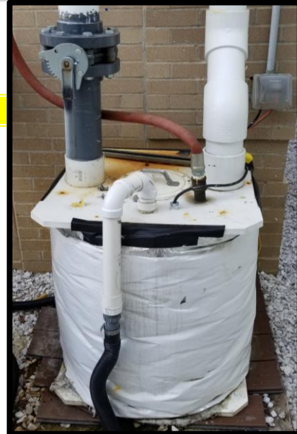
FLUE GAS FILTRATION
