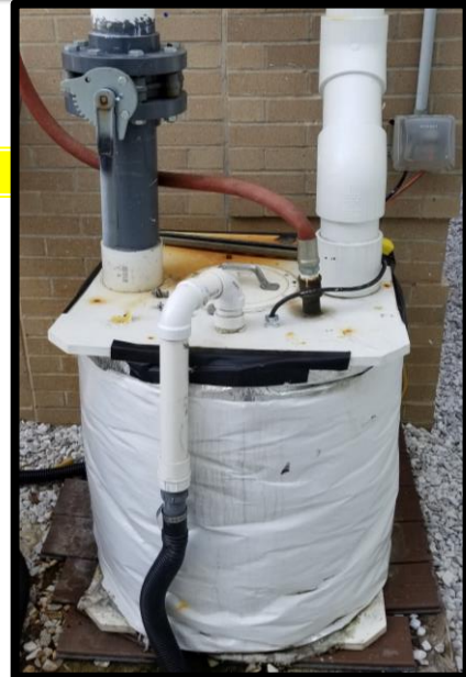
FLUE GAS FILTRATION
