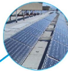
Rooftop Solar Photovoltaic (PV)
