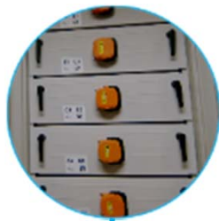
Battery Energy Storage System
